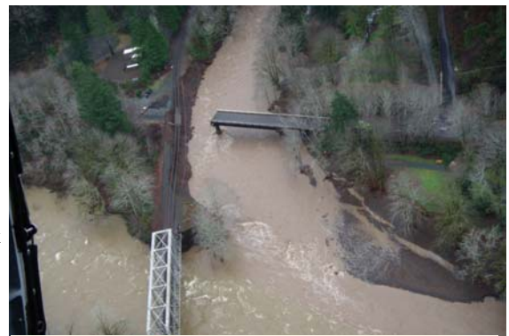
Storm damage to a co-located bridge, railroad, and fiber optic main
